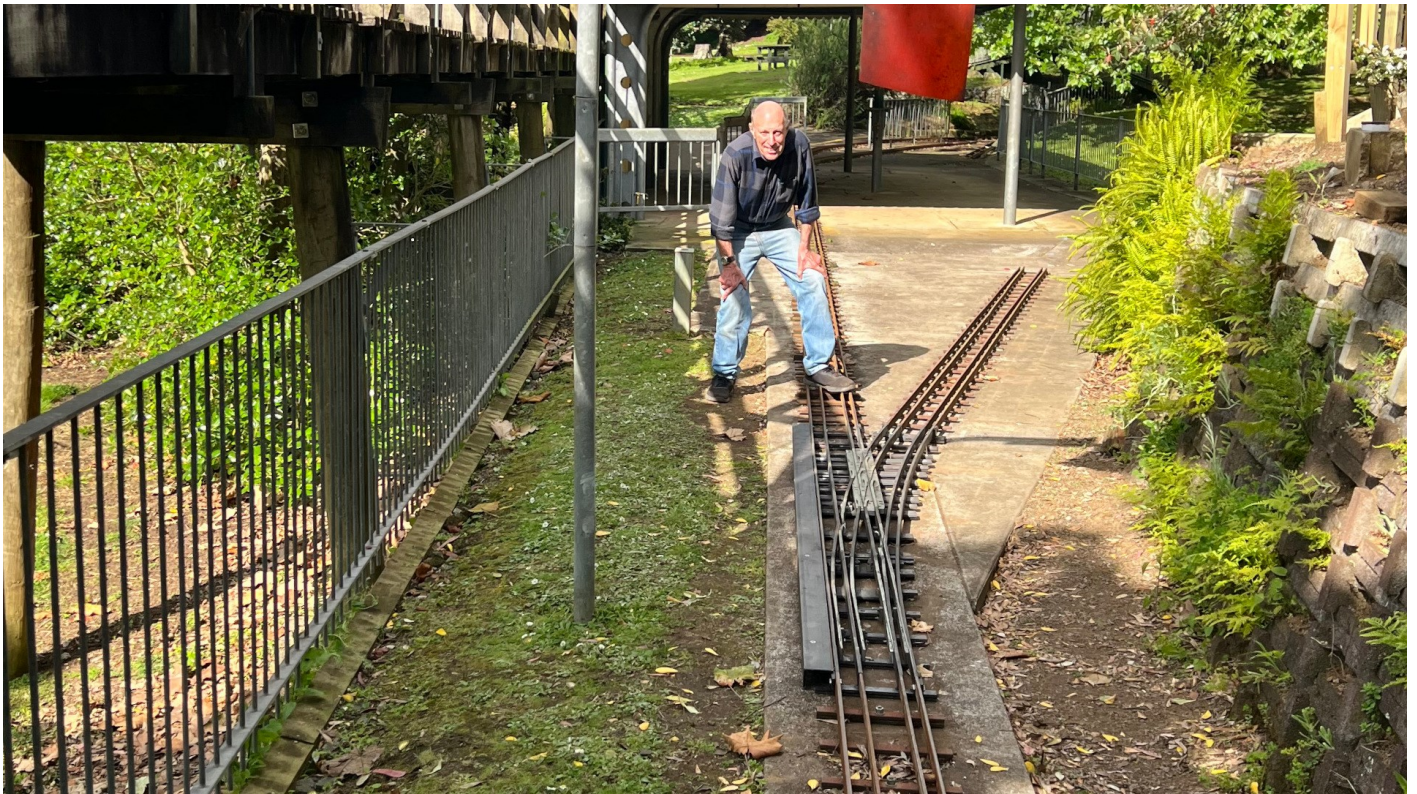
The new station points freshly installed. Mike Banks and his team have done a fantastic job on this!
