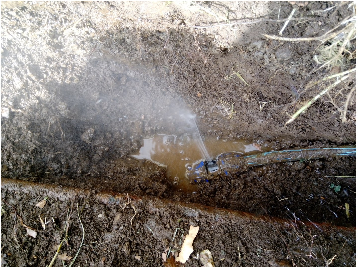
The challenge of a cracked underground fitting
