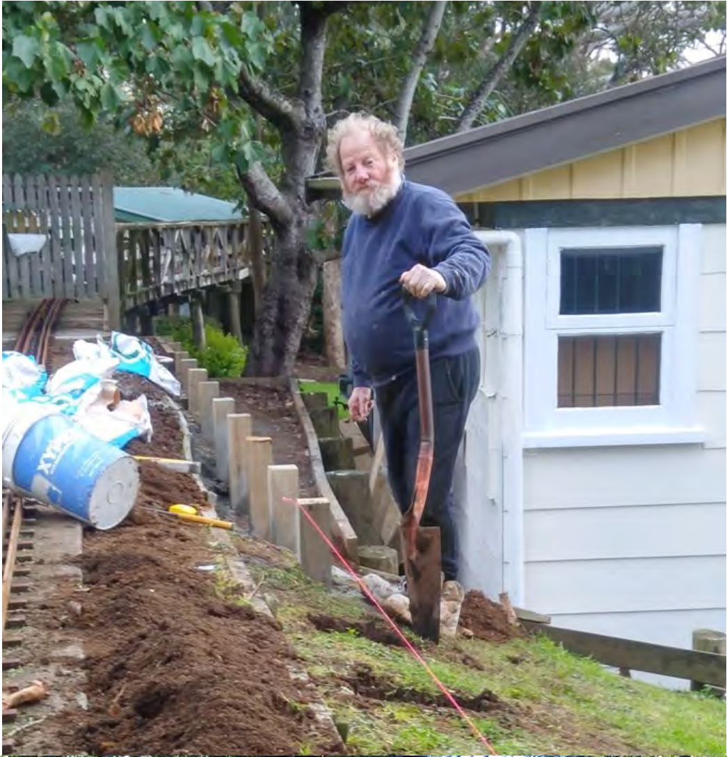
Tony Lawrence views early work in the rebuilding of the retaining wall between the two trestle bridges
